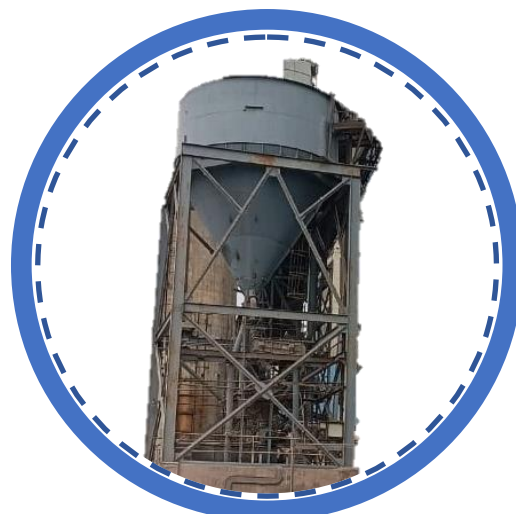
Bed ash re-cycling, with sieving machine installed. Re-cycle to bed material Bunker
