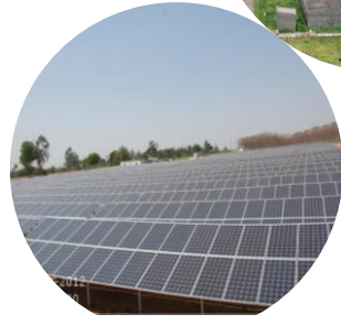
1.15MW Solar Power Plant
